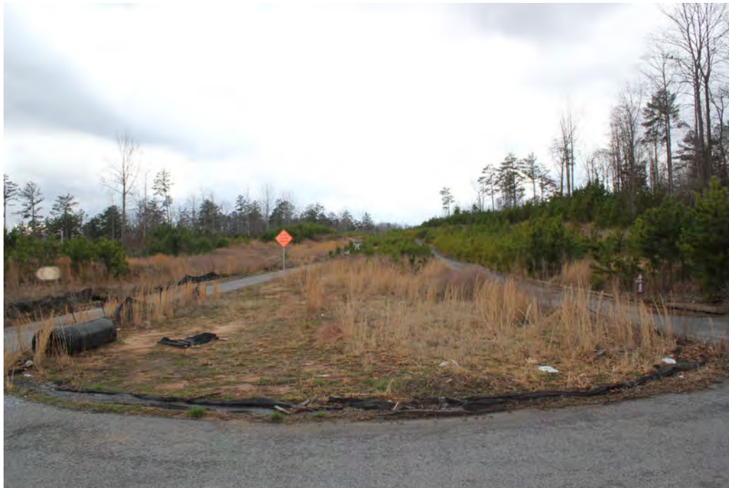
Picture 20—Unfinished Streets and Infrastructure
